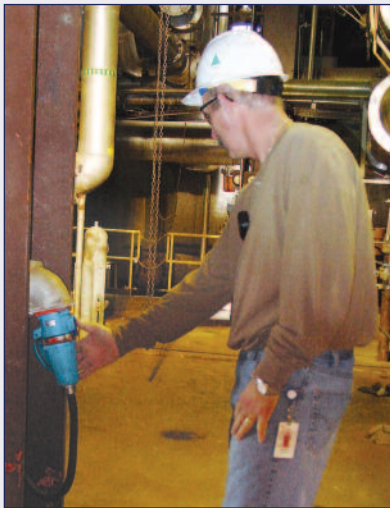
Mechanics can quickly and safely make and break electrical connections, without special PPE.
