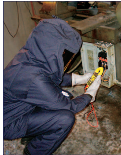
After operating the disconnect switch, a worker still needs to verify deenergization. Exposure to live parts is inevitable, so PPE is required.
